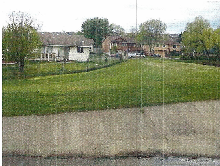
The downstream slope, as seen from the left end of the dam embankment.
