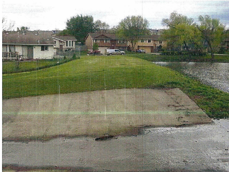
The crest of the dam, as seen from the left end of the dam embankment.
